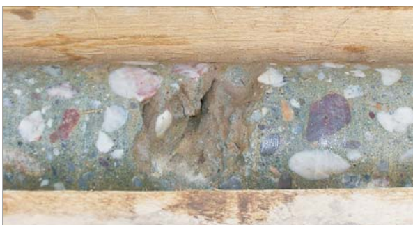
Result of core drilling for verifying the integrity test: cavity in the imperfection area
